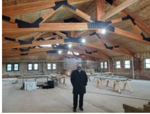
Developer David Ball stands below the new roof of Pythian Castle. Photo Credit: Sean Nestor.
